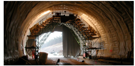
[Tunnel Application, Germany]
