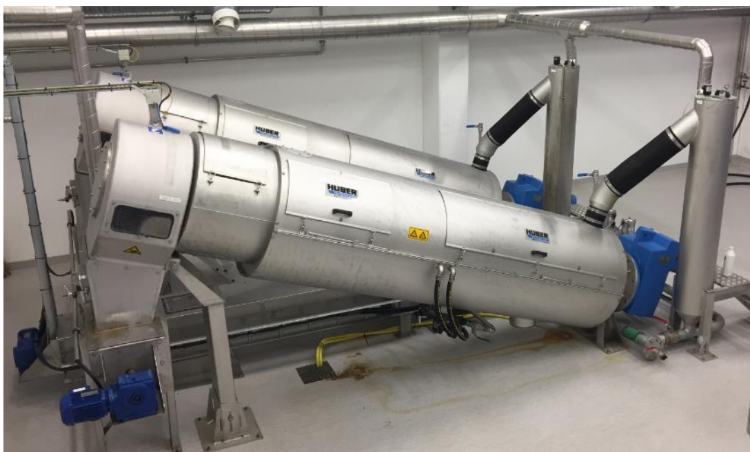
Figur 11: Skru presseser for slamavvanning, Hartevatn RA
